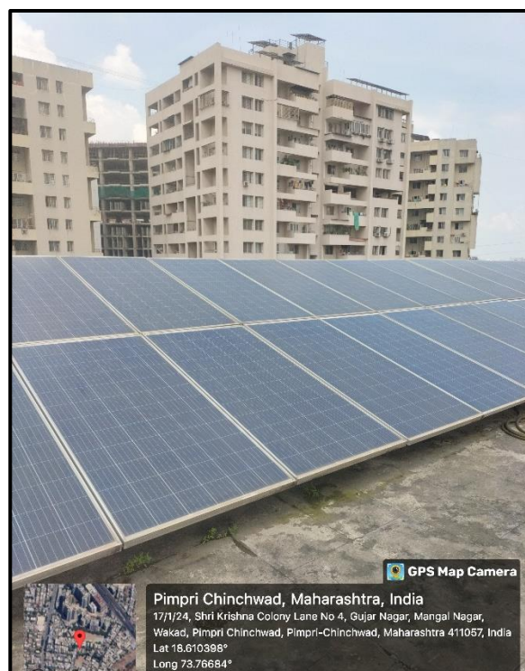
Photograph of 10 kWp Roof Top Solar PV Plant:
